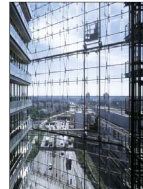
Supervision of air and driving rain leakage testing of curtain wall systems
