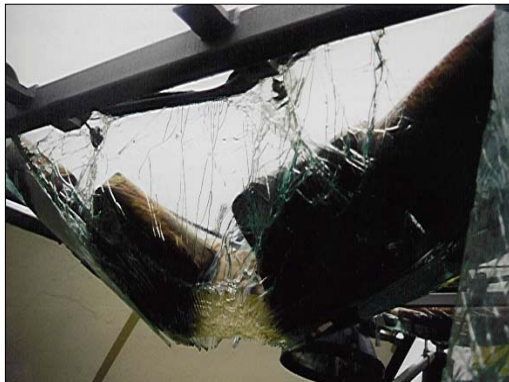
Post breakage behaviour of horizontal glazing systems
